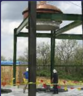
LEFT: Threading the needle with a copper hood. Note the calandria peeking out of the floor.
